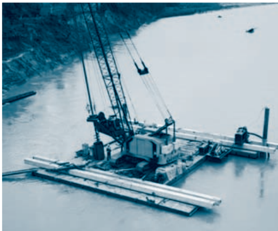
Crane-mounted drill using an "H" shaped assembly to permit work within restricted reach conditions.
