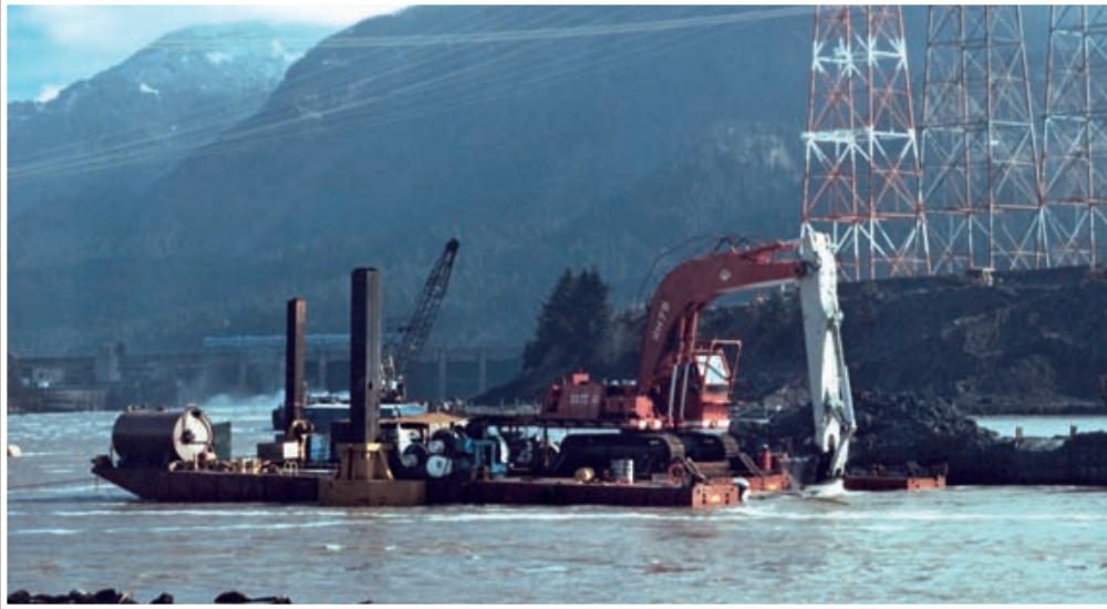
An 8-cubic yard hydraulic excavator, supported on a 60-ft. x 120-ft. x 7-ft. assembly, dredging to minus 35 ft.
