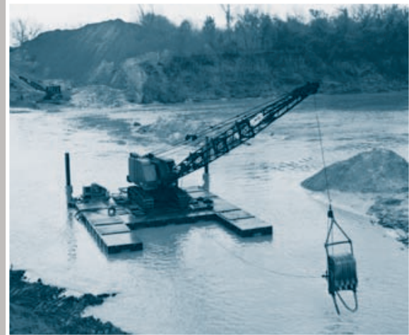
Series H-50 spud barge allows 1-cubic yard dragline to operate in very shallow water.
