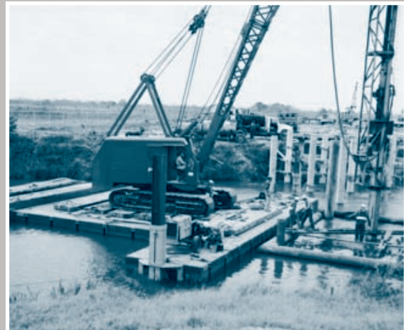
65-ton crane on Series S-50 equipment driving piling in a narrow canal.
